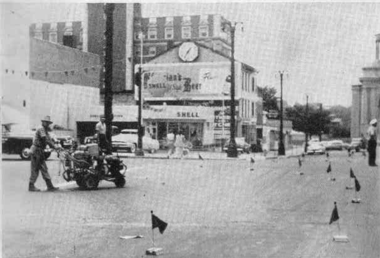
TRAFFIC LANES MUST BE PAINTED
