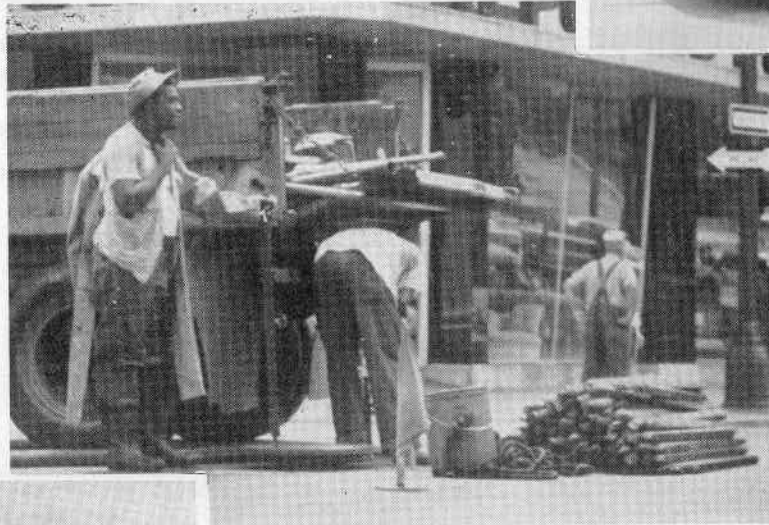
SEWERS MUST BE CLEANED
