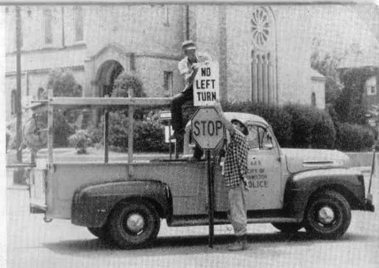
SIGNS MUST BE INSTALLED
